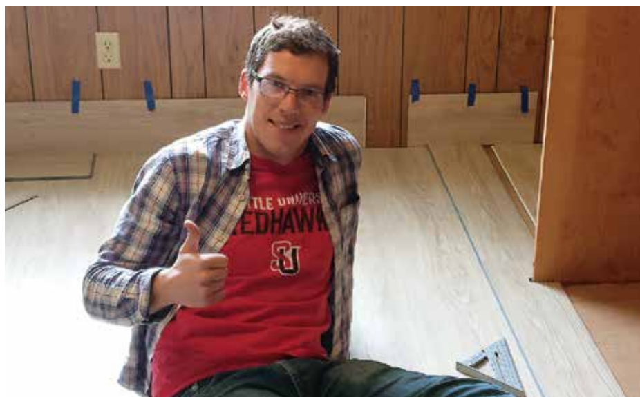
James Millikan, SJ, completing a kitchen remodel and new floors in Newtok, Alaska.
